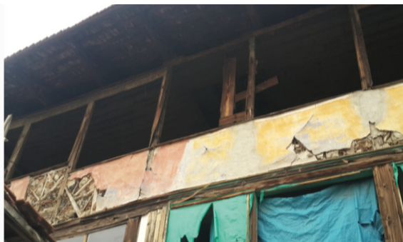
Figure 10. Physically deteriorated building elements
