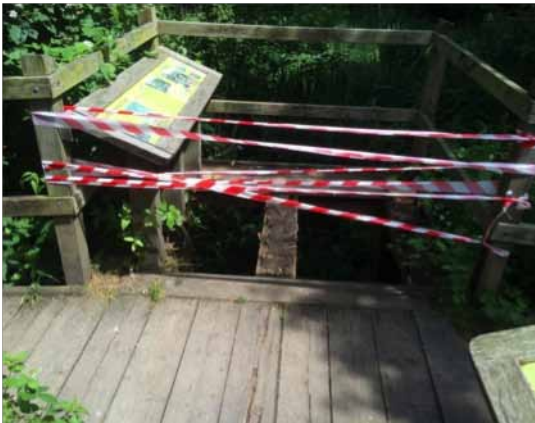
Old bridge rotten and vandalised
