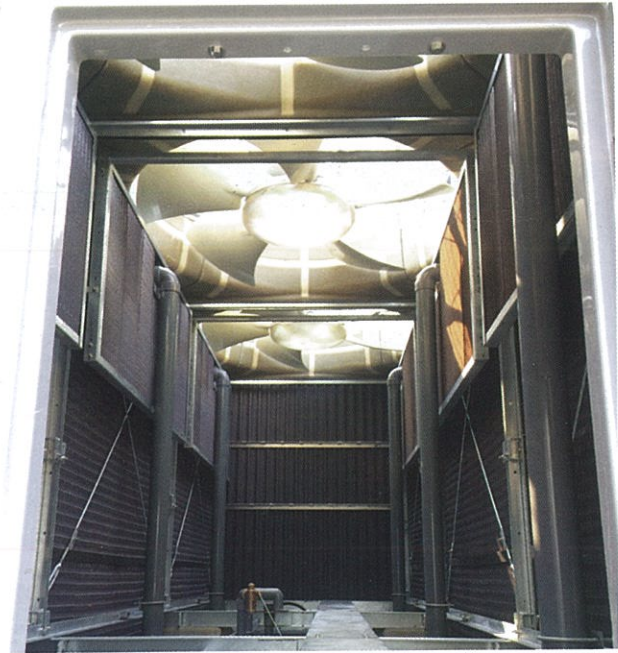
The Kaer Water plant at Orchard Towers, after the upgrading
