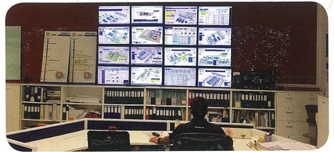
The K-RealTime Broadcast Centre monitors, controls and optimises over 40 air-conditioning systems in Singapore, Malaysia and Indonesia.
