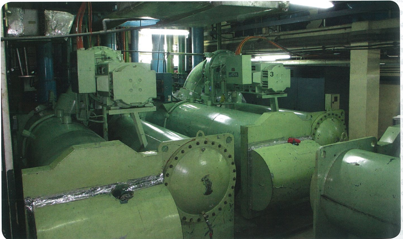
The Orchard Towers chiller plant in 2013
