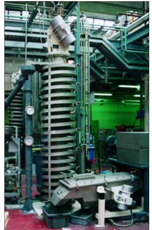
Fig. 5 Cooling spiral conveyor with a screening machine in a plastics factory
