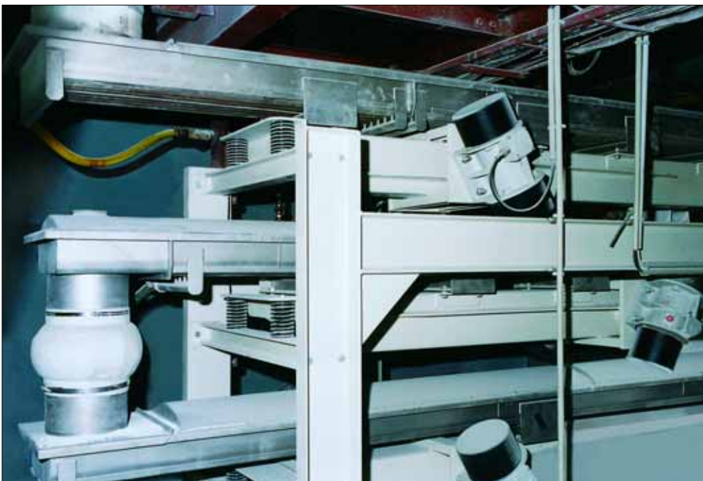
Fig. 6 Three cooling trough conveyors arranged in a cascade
