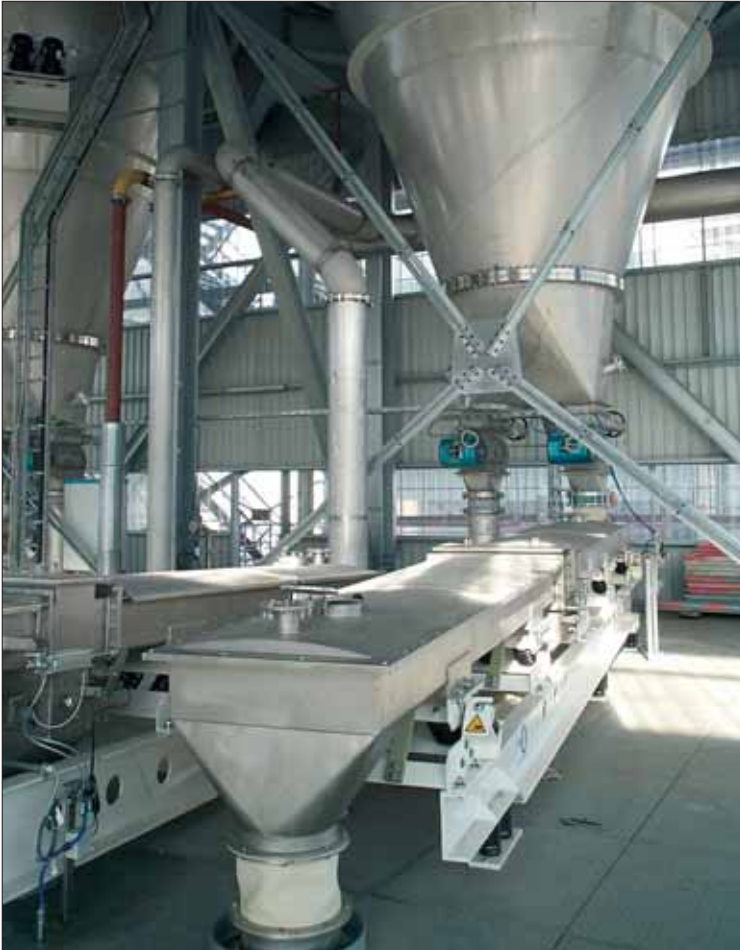
Fig. 30 Discharging from silos
