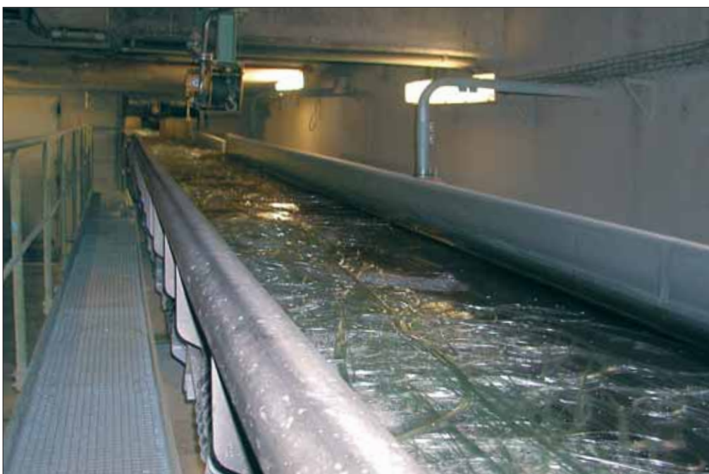
Fig. 17 Part of a 200 m long conveyor system for glass fibers
