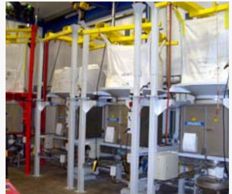
Big-Bag Emptying, with containment
