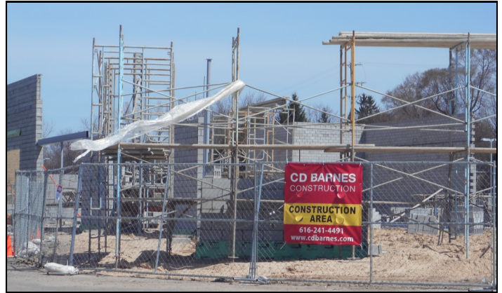
New retail space is under construction between Fifth Third Bank and Leigh's
