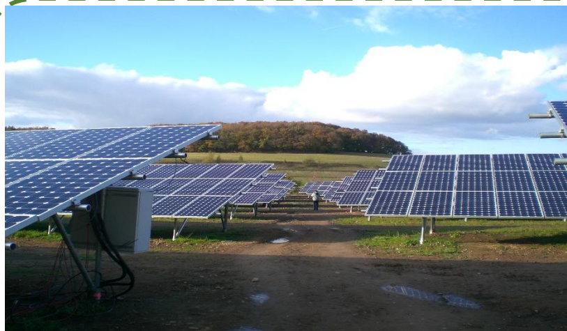
15MW, UK Chelvest Energy Park
