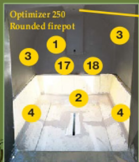
Extensive amount of heavy-duty pre-cast heat-treated refractory brick
