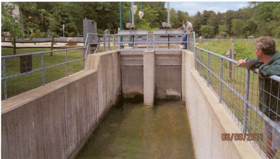
Slide Gates - Upstream (0009300609201154)
