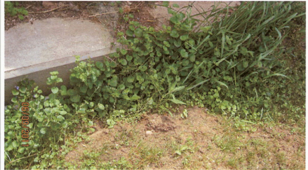
Toe Drain Erosion Area (0009300609201153)
