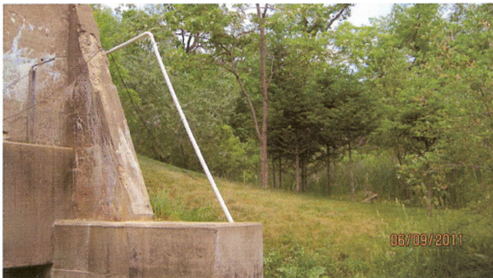
D/S Left Side Embankment (0009300609201134)
