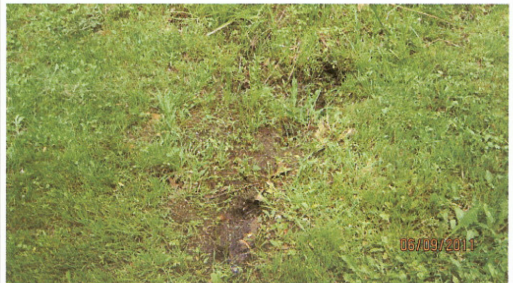
Minor Seepage Area D/S Left Side (0009300609201143)
