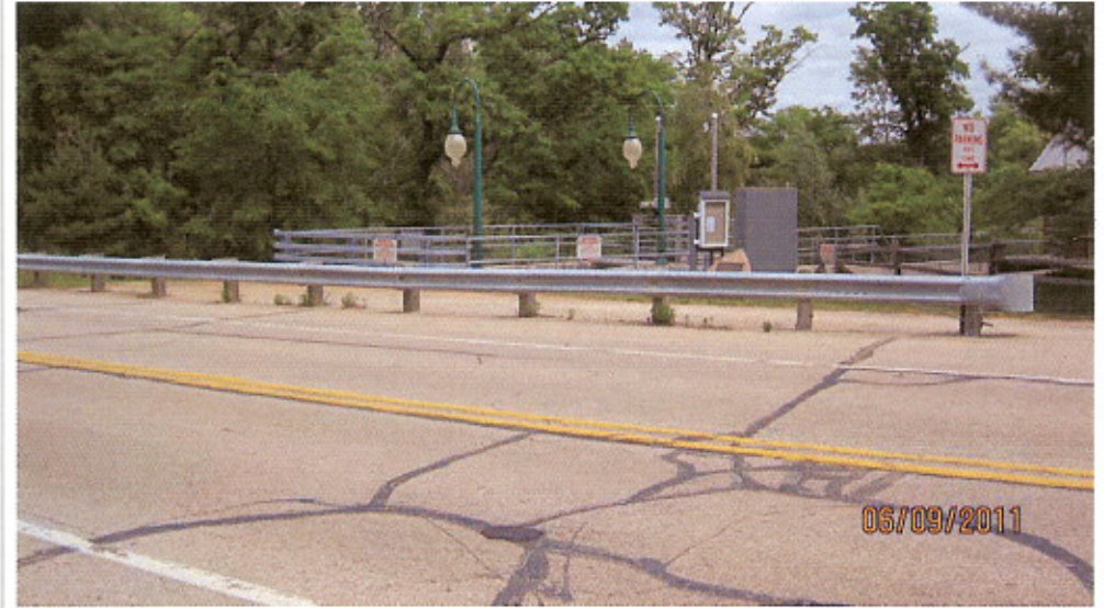
Flume / Gate Controls (0009300609201158)
