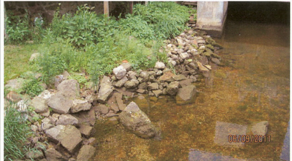
D/S Right Tailwater Rip Rap (0009300609201138)
