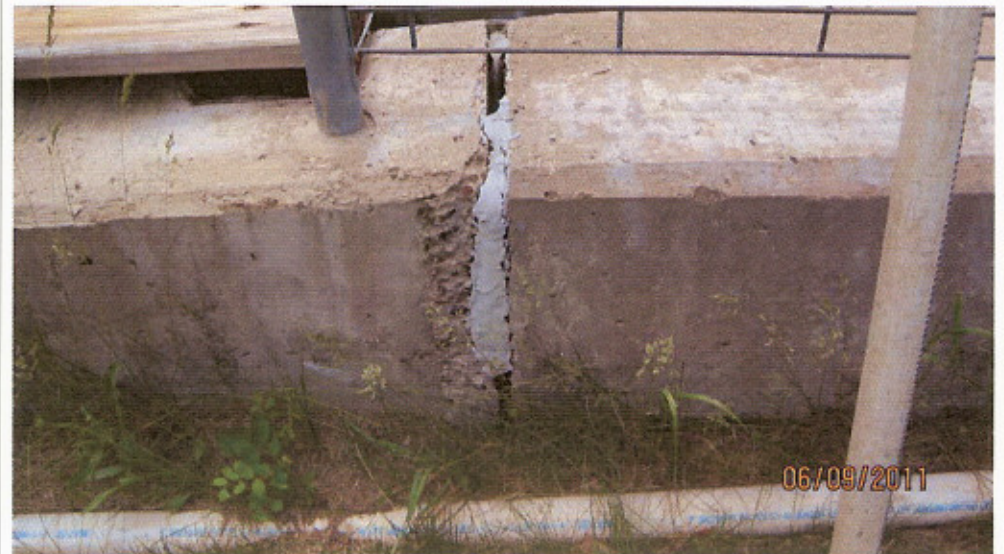
Flume Construction Joint (0009300609201156)
